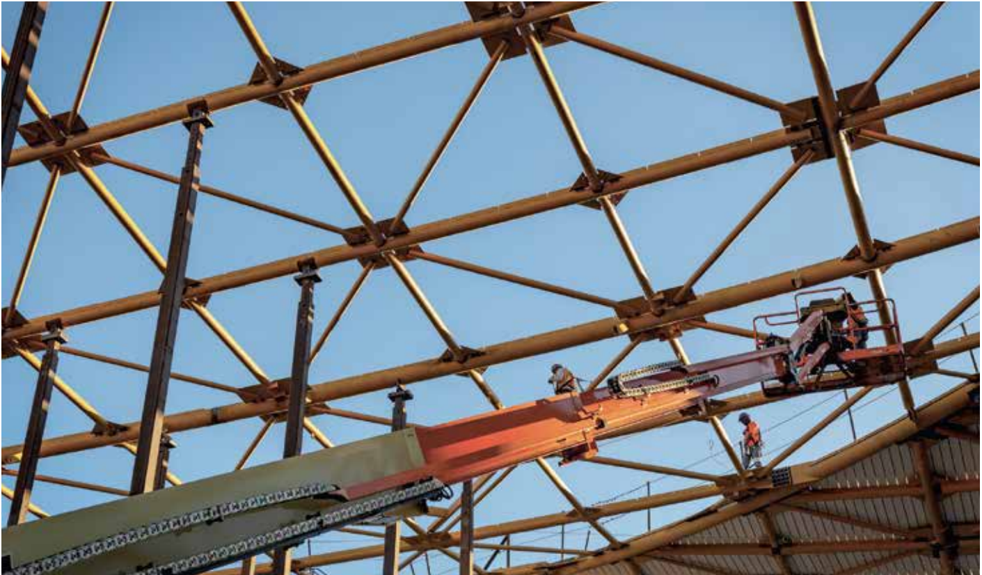
Above: “Tube net” steel is in place as work on the roof is advanced at Charleston East.
