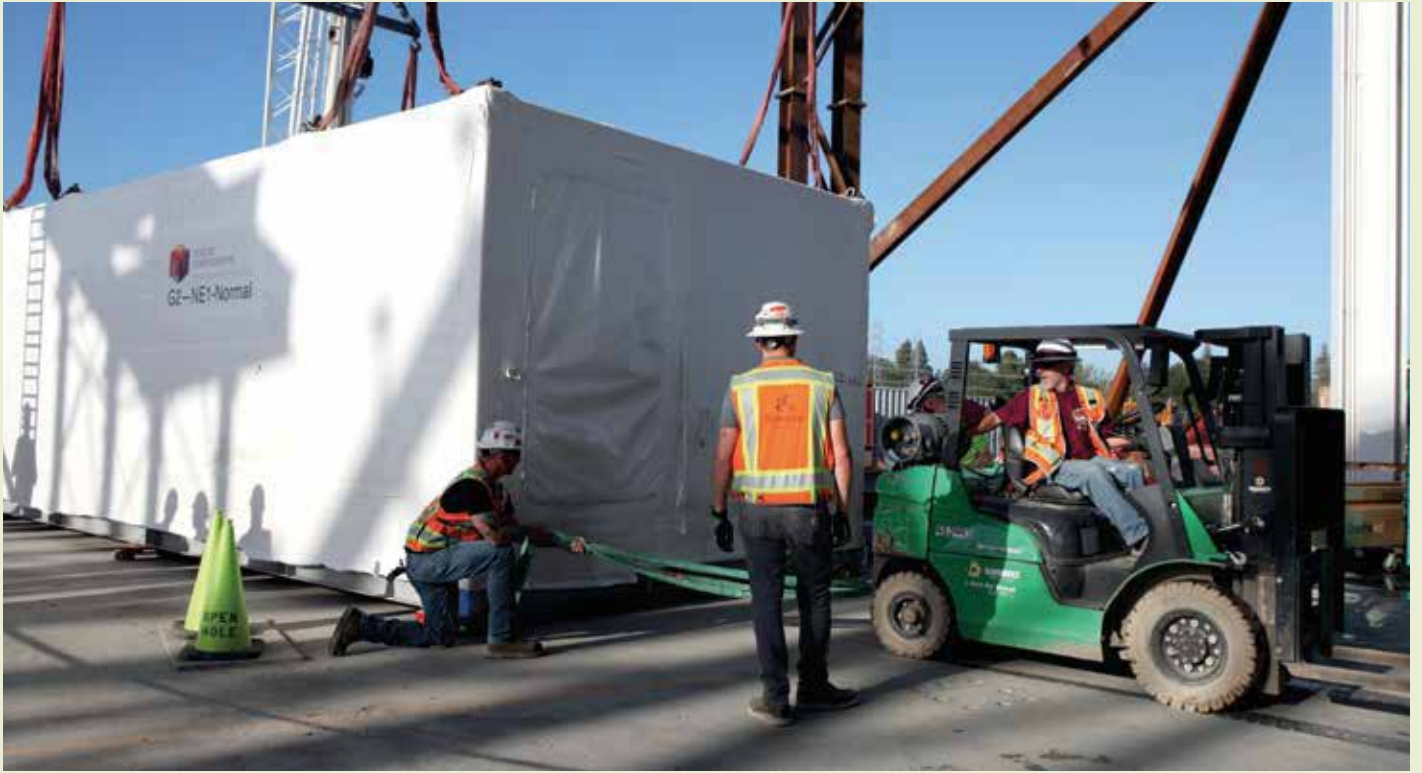
Prefabricated modular units arrive at Bay View and are readied for stacking as part of the short-term corporate accommodations.
