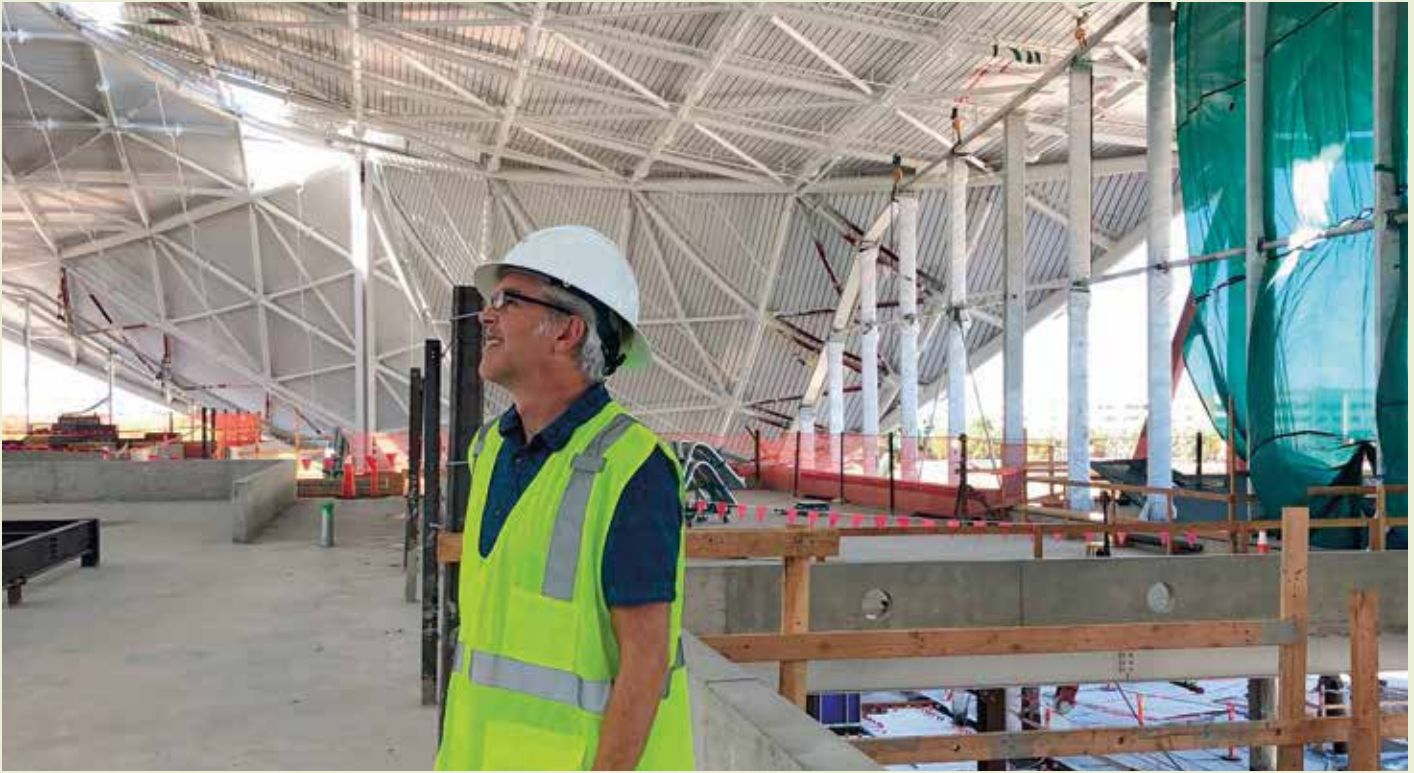
Eric Solrain of Integral Group surveys construction progress on the upper level of Bay View prior to installation of MEP systems.
